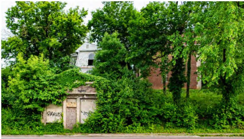
Some properties along West Broad Street are overgrown, abandoned, and deteriorating. This retail space near Lechner & Broad was home to a confectionery, a carpenter, and a florist shop, but was vacant by the 1970s.
