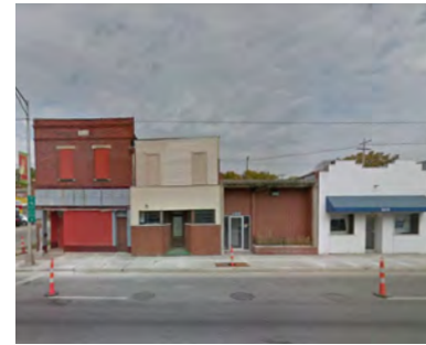
A section of deteriorating buildings on W. Broad at the intersection with Eureka Avenue.
